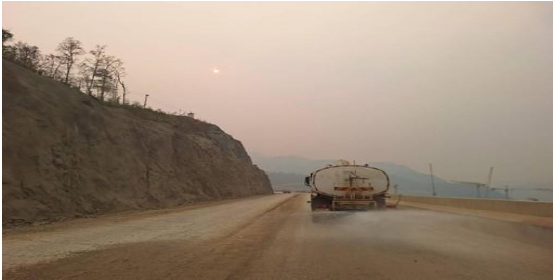
Water Recycling Project from a Batching Plant Project
